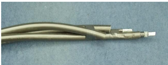
Figure 10: Covered Conductors Morne Diablo
