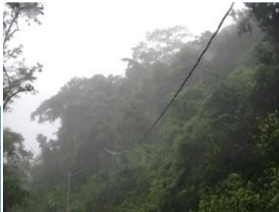
Figure 11: Covered Conductors being used in Morne Diablo
